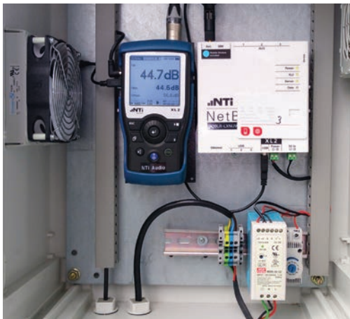
Interior of a weatherproof Enclosure
