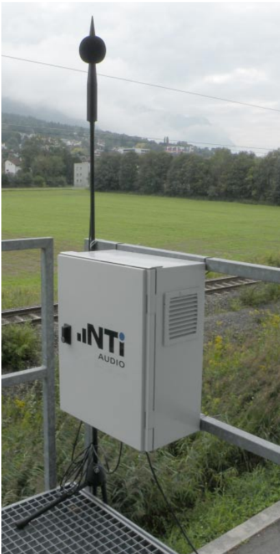
Noise Monitoring Terminal with outdoor mic mounted on tripod
