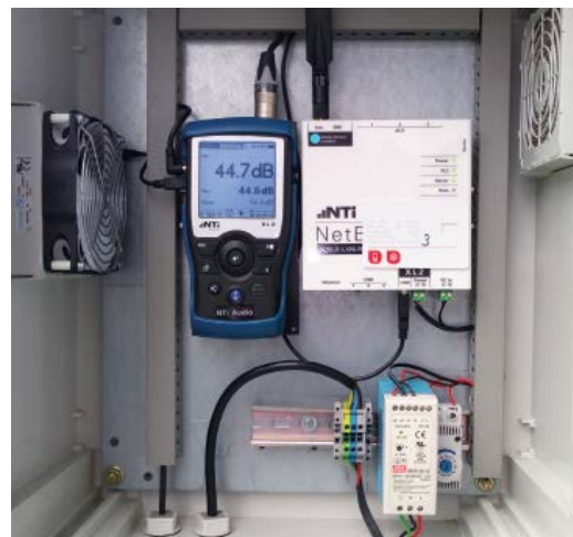
Station de surveillance autonome
